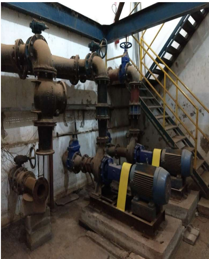
(a) Bombas KSB Megaflow 150-315 de 150 m 3 /s
